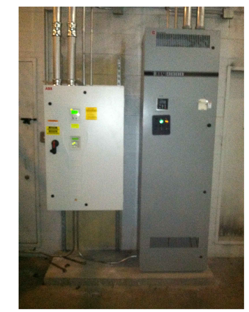
PHOTO: VFD FOR AHU-4 (TO REMAIN) AND AHU-3 TO BE REPLACED
