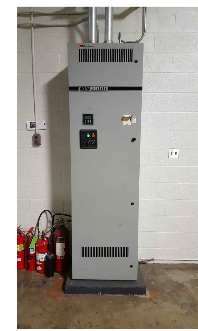
PHOTO: VFD FOR AHU-2 TO BE REPLACED
